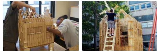
Figure 6 Laser cut model at 1'' = 1'0'' (a), the same information used to build the final house (b) constructed exclusively of \frac{3}{4}'' plywood with studs and furniture.
